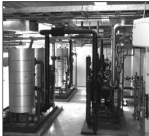
Ozone preparation room
