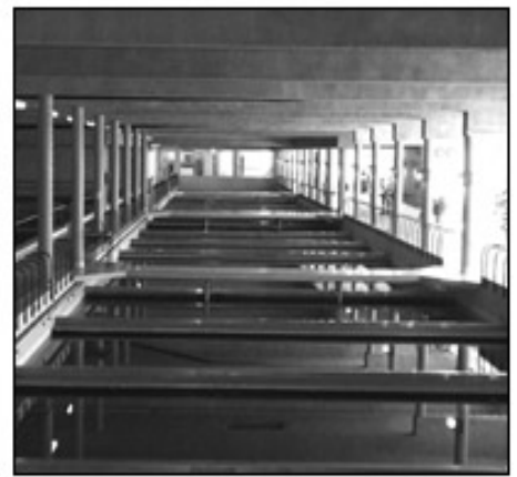
Water filtration room
