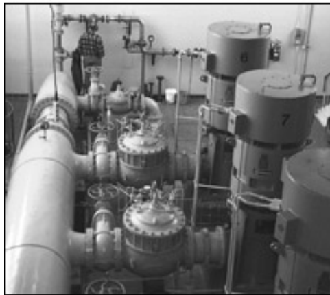
Treated water pumping room
