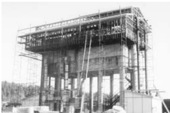
Construction of the water aeration tower and headtank at the Mactaquac Fish Culture Station in the mid 1960s - photo by Phil Hubley.
