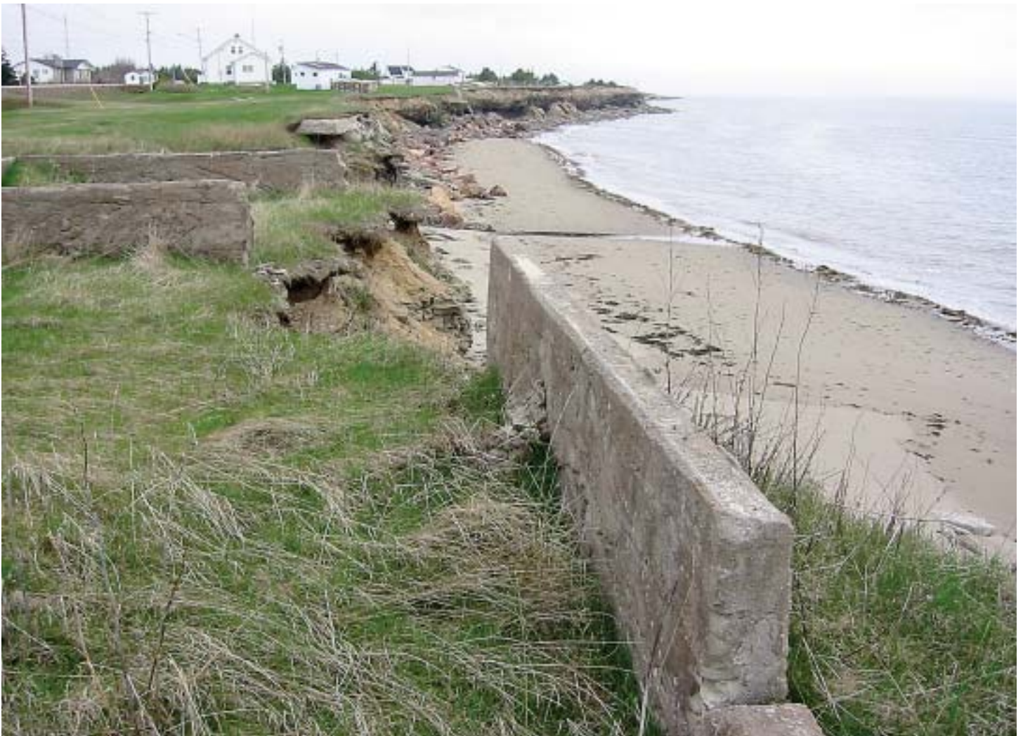
Abandoned and partly collapsed foundations attest to rapid erosion of low cliffs at Cap Lumière, NB. Other homes and businesses along this coast, including those in the background, are at risk from accelerated coastal erosion resulting from rising sea levels and other impacts of climate warming.
