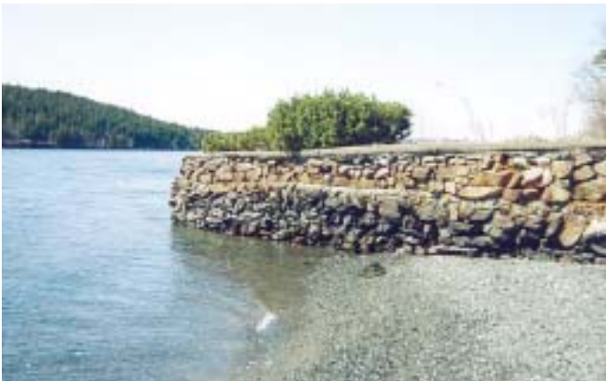
Slope altered due to infilling in the intertidal zone.
