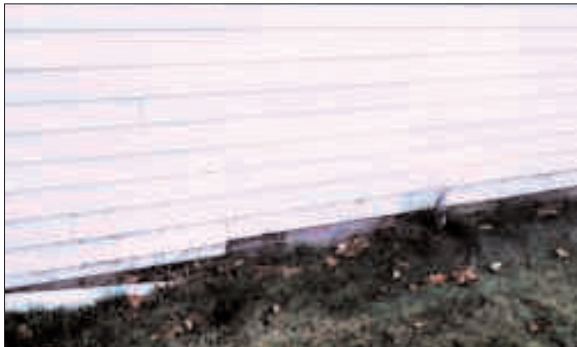
Exterior: vents too close to grade
