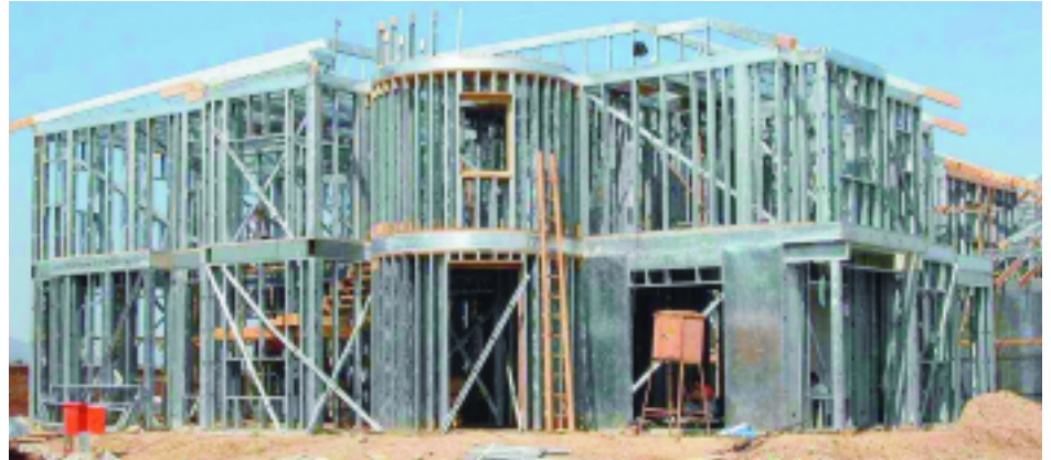
Davey International's lightweight steel frame technology used in the construction of North American-style luxury homes north of Beijing
