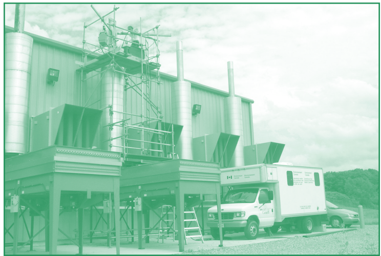
A specially equipped truck from Environment Canada's Environmental Technology Centre tests emissions from a reciprocating engine that burns landfill gas to generate electrical energy.
