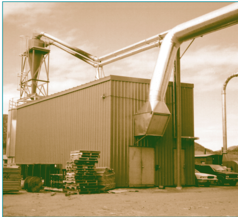
Building housing biomass unit (front view) – Above the building a set of pipes carries sanding dust from the baghouse to the silo at the rear. The large pipe coming from the front of the building is the heat duct pipe carrying warm air to the production facility. The spill vent, which is used on hot days, can be found near the bend where the heating duct goes upward.
