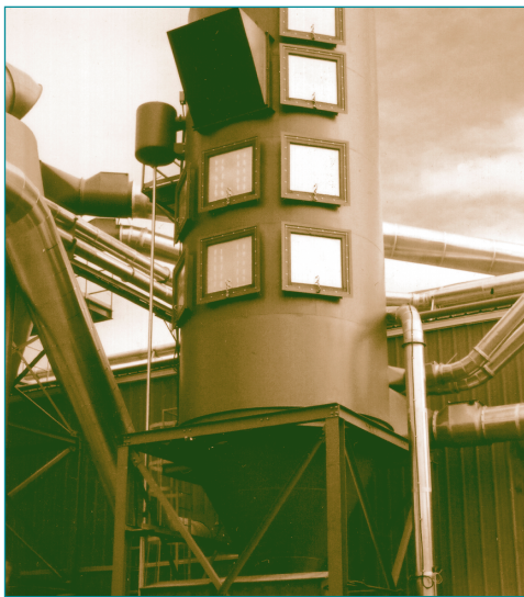
Baghouse – the baghouse collects the dust produced by the sanders in the production plant. The large pipe coming in from upper left and curving down and past the baghouse and into the building in the background is the heating duct carrying warm air from the biomass unit. The heating duct is approximately 1 m (3 ft.) in diameter.
