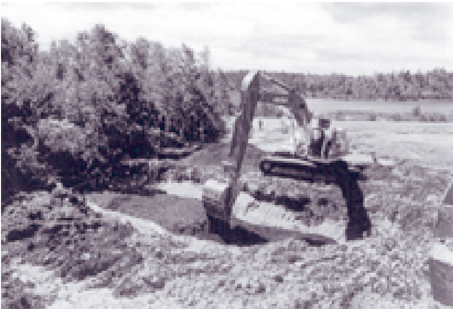
Installation of a permeable reactive barrier for the treatment of acid mine drainage, near Sudbury, Ontario.
