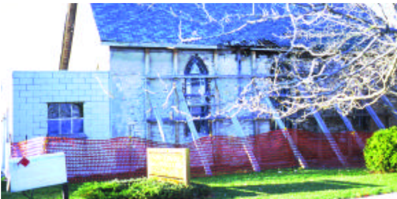
Before and after photos of emergency conservation work at the Nazrey African Episcopal Church in Amherstburg, Ontario
