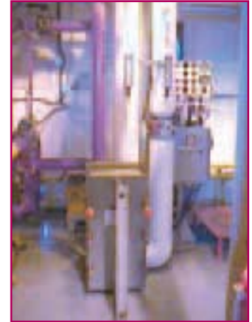
Main jacket water heat exchanger
