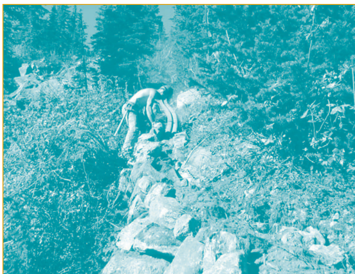
Figure 14. High-density polyethylene (HDPE) penstock being buried in a steep hill (photo courtesy of Thompson and Howe Energy Systems Inc.)
