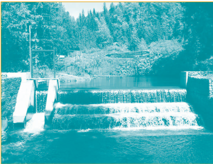
Figure 10. Intake of micro-hydropower system in Seaton Creek, British Columbia (photo courtesy of Homestead Hydro Systems)
