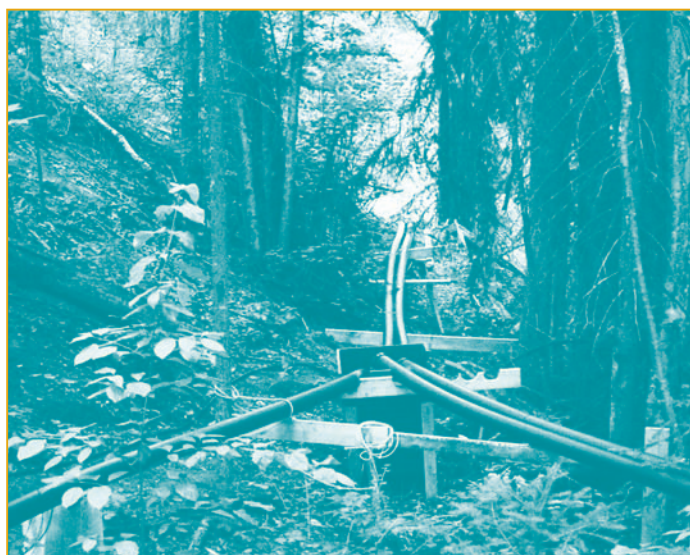
Figure 15. Double 10-cm (4-in.) HDPE penstock pipe for an 8-kW system
