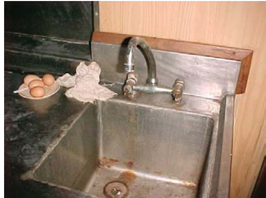
Unclean galley/No control valve for faucet
