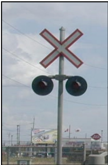
Figure 2.3 Automated warnings: crossbuck sign with flashing lights.
