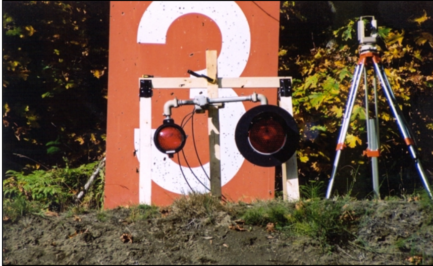
Figure 35 Mounting Arrangement for New Incandescent Modules
