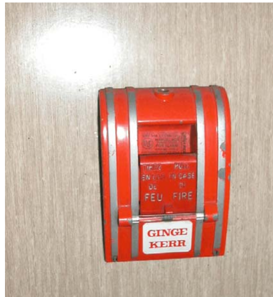
Photo 4. Typical manual pull station
