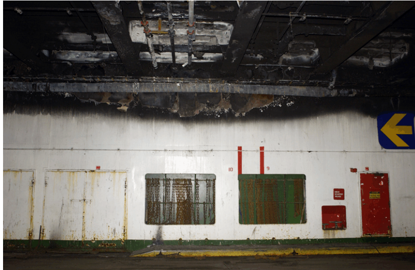
Photo 2. Damage to deckhead
