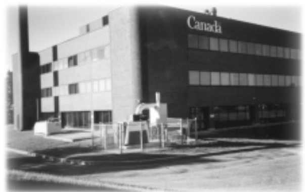
A microturbine is producing electricity for a Health Canada lab in Toronto. Small on-site electricity generation makes use of waste heat and reduces carbon dioxide emissions.
