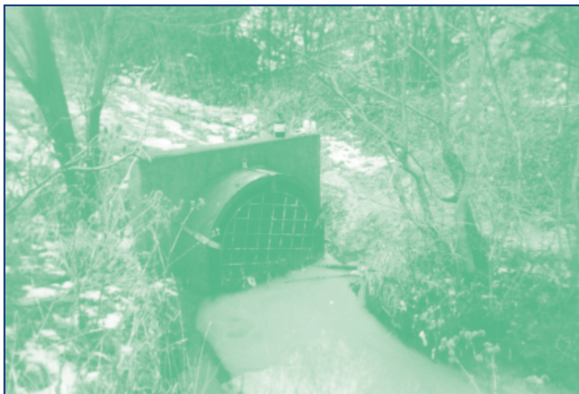
The outflow from this combined sewer located in an older residential area of Hamilton, Ontario, discharges into a small creek that flows into the Cootes Paradise area of Hamilton Harbour.
