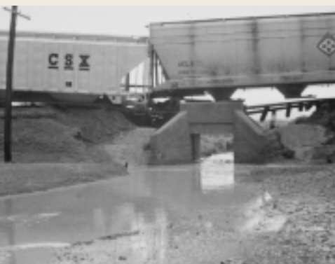
Erosion damage to rail line
