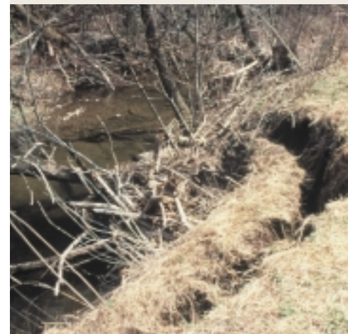
River bank erosion
