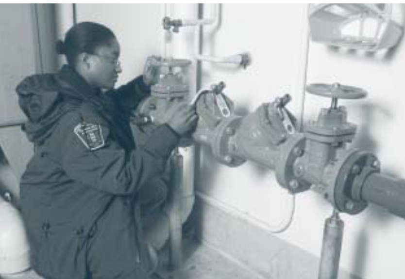
MOE inspector checking back-flow preventer and valve integrity
