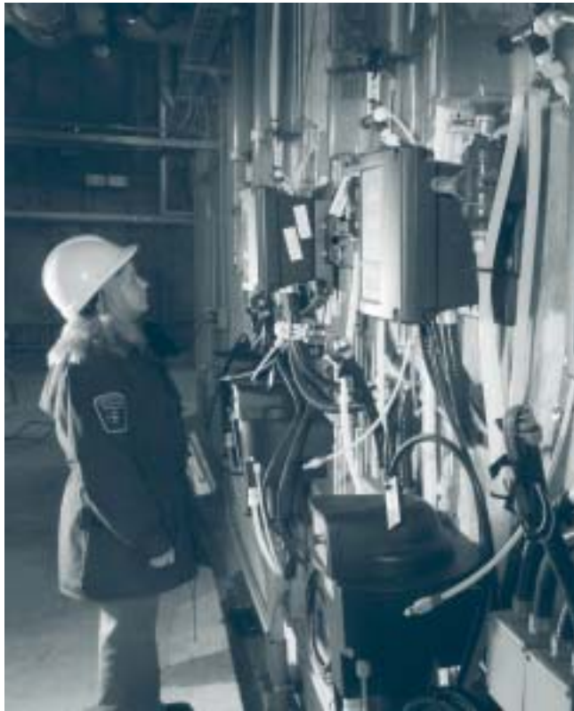
Inspecting digital display of continuous monitoring equipment
