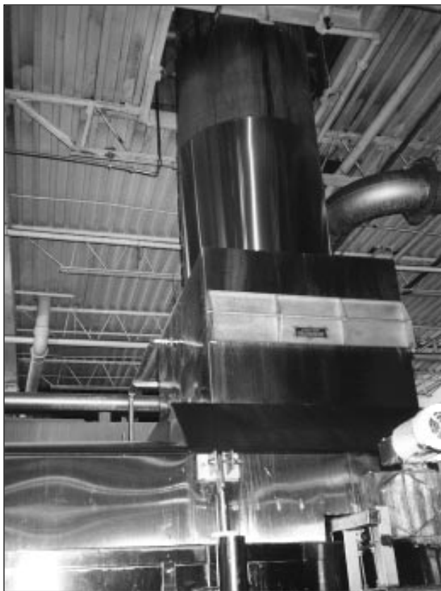
The final report recommended the installation of heat recovery equipment in the exhaust of potato chip flyers.
