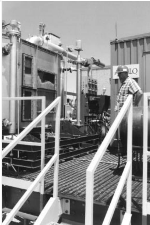
Scrubber in operation
