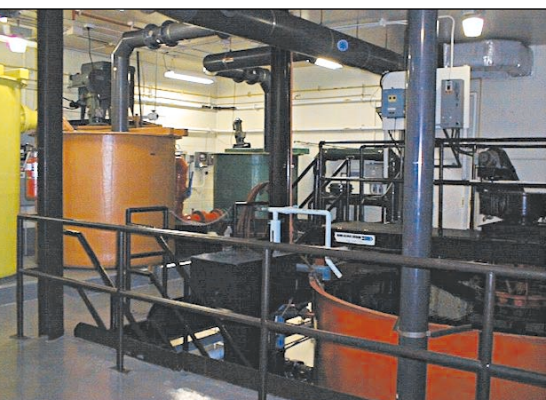
Interior of the arsenic treatment plant.
