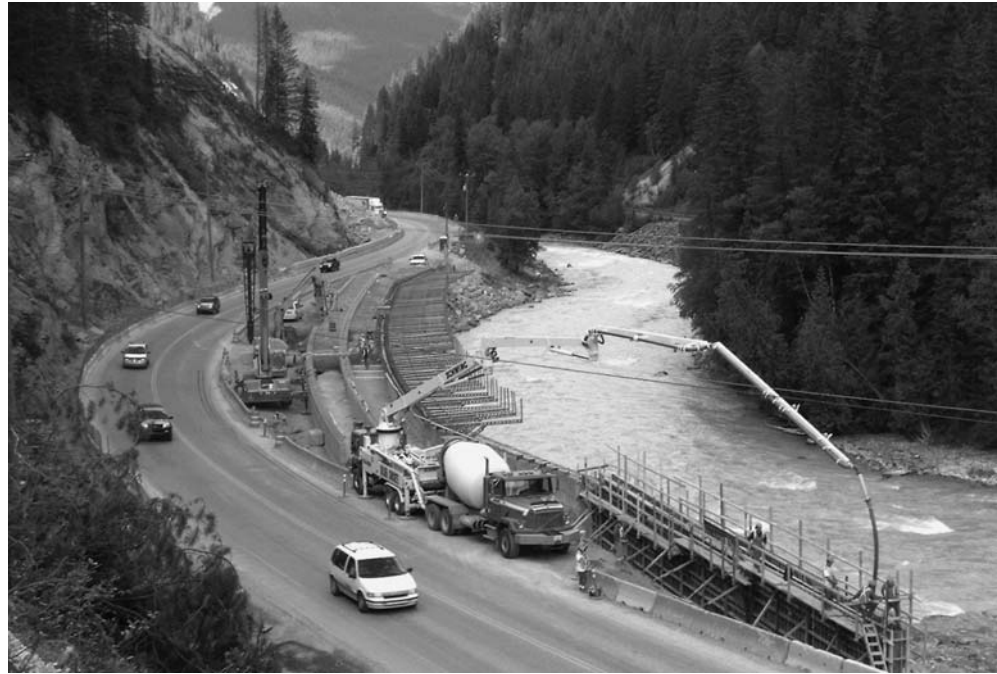
Pouring of retaining wall on the cantilever structure between Yoho Bridge and the Rafters Pullout
