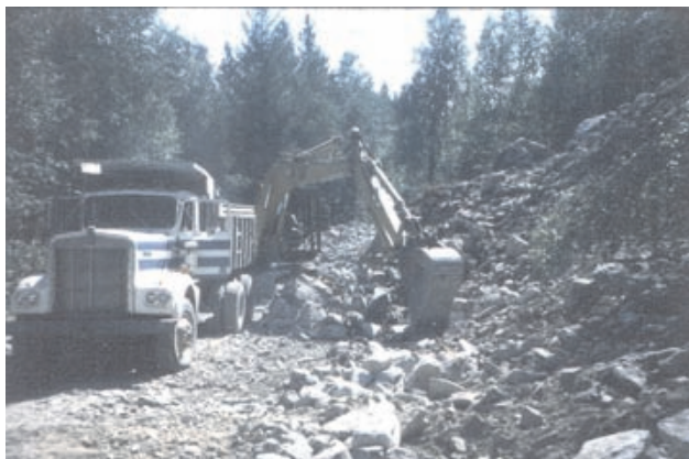
Photo 2. Active mining of the colluvium along Lillooet Forest Service Road, in the upper Lillooet River Valley. Material here is being used to armor river banks (rip-rap) along reaches where erosion threatens the logging road. Other locations provide aggregate for road base and diking material.
