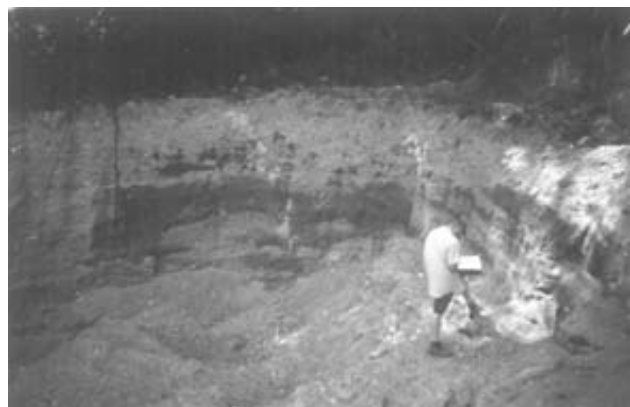
Photo 1. An example of a small borrow pit located near the town of Gibsons where material is being extracted for road construction on private land.
