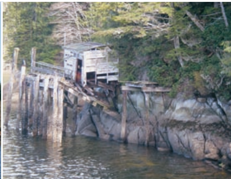
Goose Bay – Former fuel storage area close to collapsing
