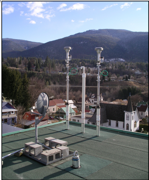
Figure 4 – TEOM continuous samplers for PM 10 , PM 2.5 , and ozone atop the current government building. These were installed in 2005.
