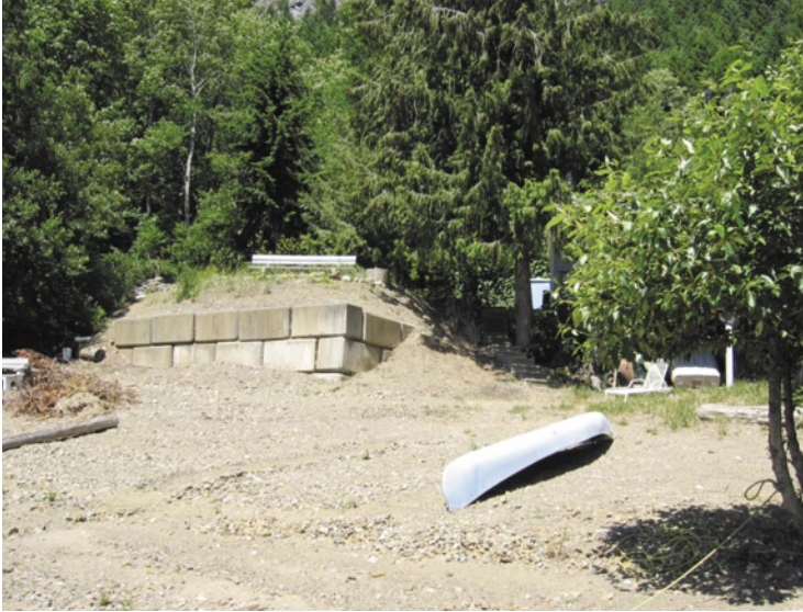
Figure 12. A terrace built out onto an otherwise stable beach. The shoreline erosion rating is Low, but the terrace itself presents a much higher erosion hazard, mitigated in this case by concrete lock-blocks.
