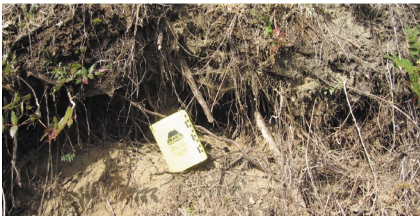
Figure 1 Unconsolidated soil is highly vulnerable to both wave action and drawdown.
