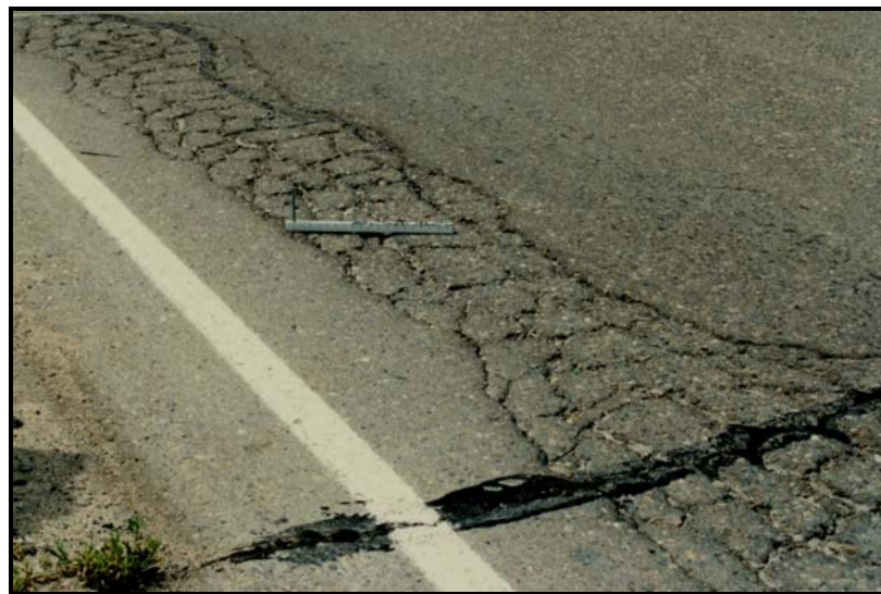
Figure 4 - High Severity LWP (alligator cracking)
