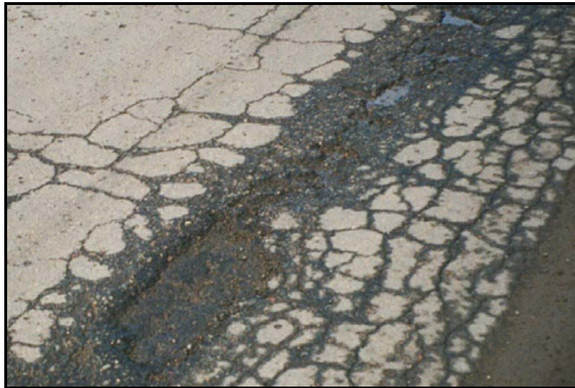
Figure 38 - High Severity POT (AC with pieces broken out)
