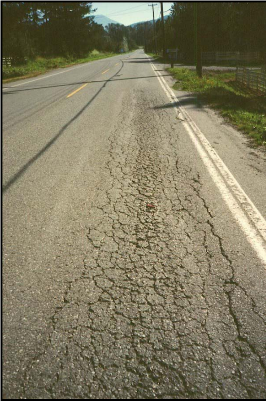
Figure 23 - High Severity AC (spalling and frequent density)
