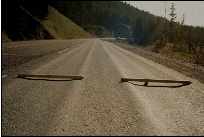
Figure 27 - High Severity RUT with transverse displacement
