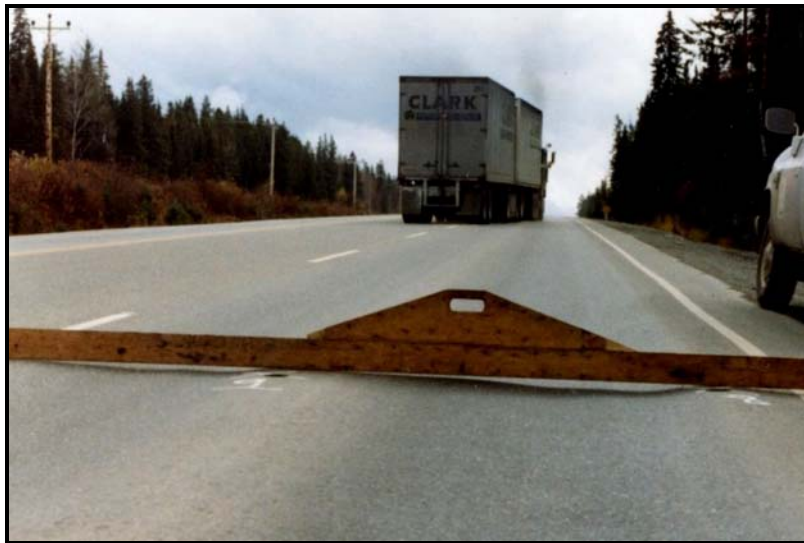
Figure 28 - High Severity RUT
