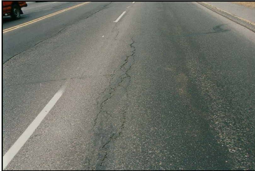
Figure 3 - High Severity LWP (multiple cracks)
