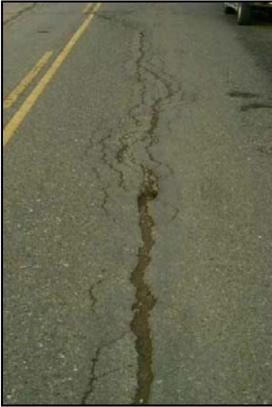
Figure 19 - High Severity MLC (multiple and alligator cracking)
