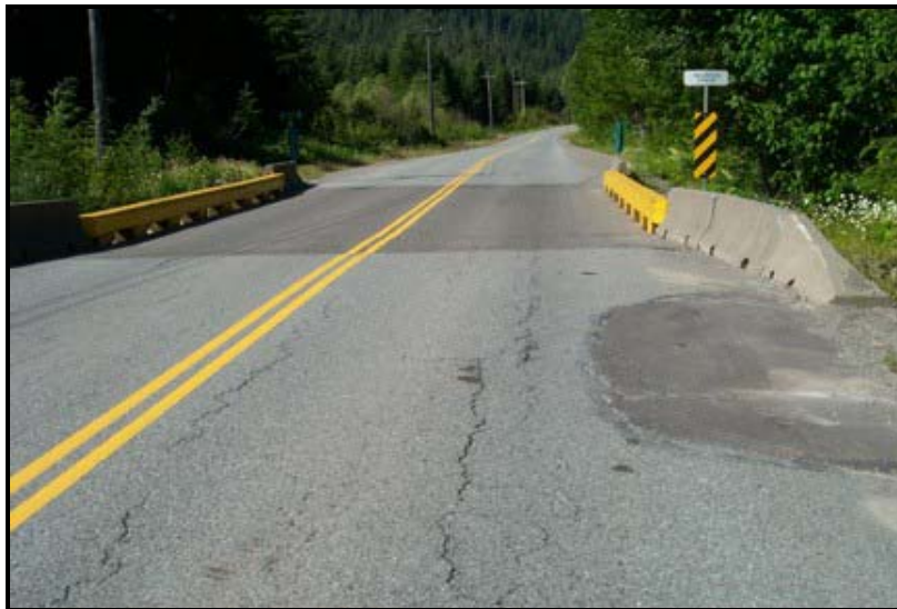
Figure 32 - Moderate Severity DST (example of pavement edge settlement)
