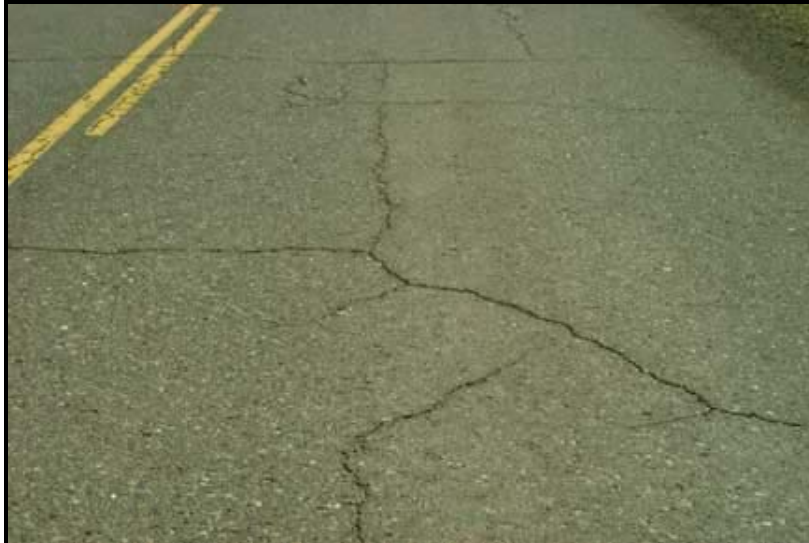
Figure 18 - Moderate Severity MLC (with secondary transverse cracking)
