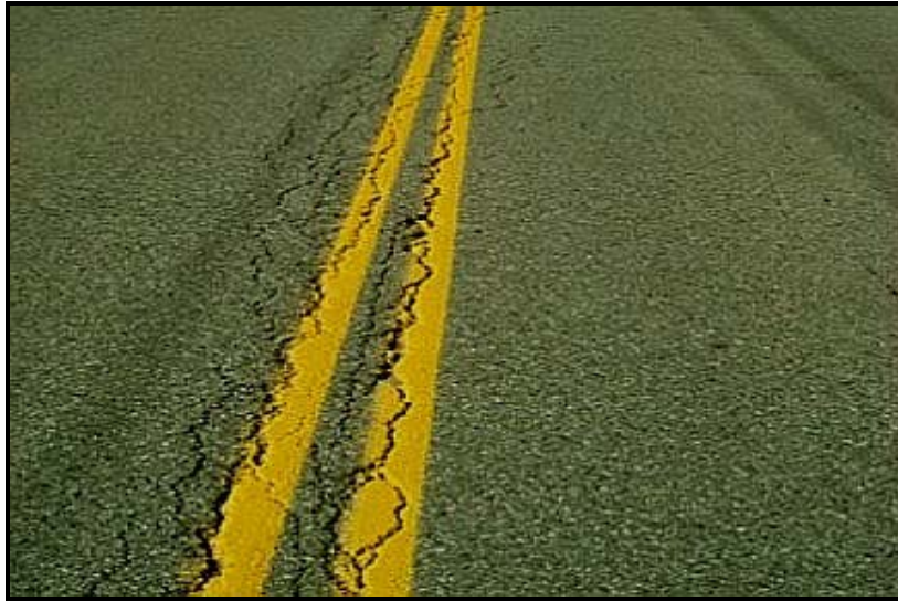
Figure 7 - High Severity LJC (multiple cracks)
