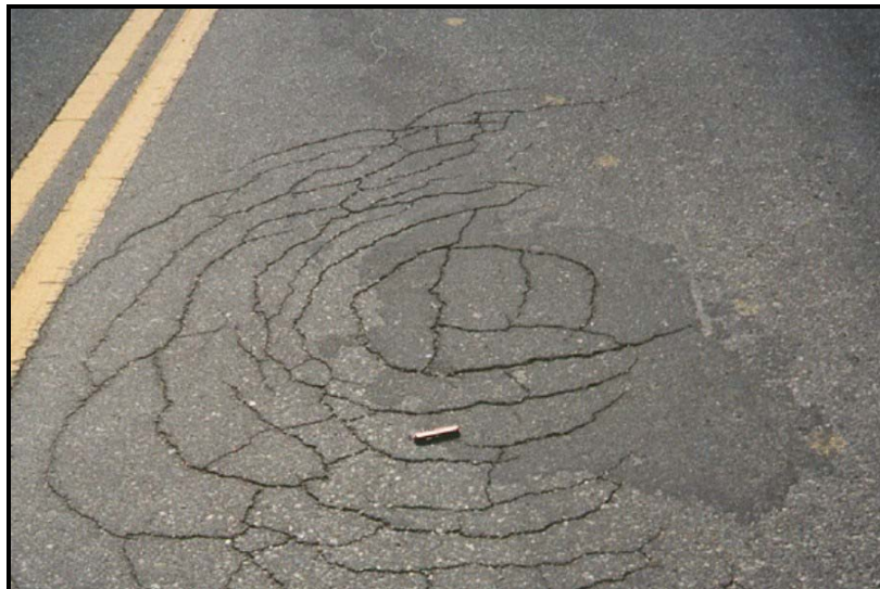
Figure 22 - Moderate Severity AC (localized failure)
