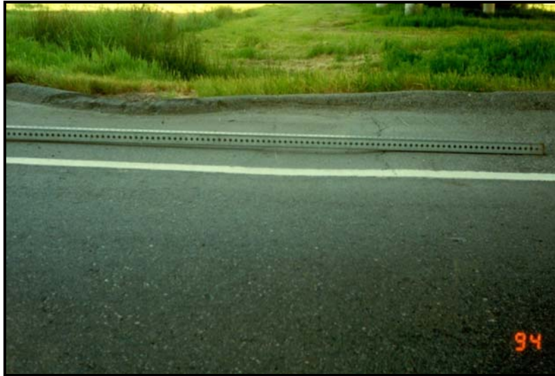
Figure 31 - Moderate Severity DST (resulting from differential settlement)
