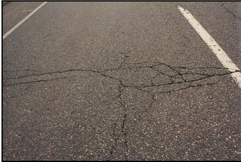
Figure 21 - Moderate Severity AC (progressed from multiple cracks)
