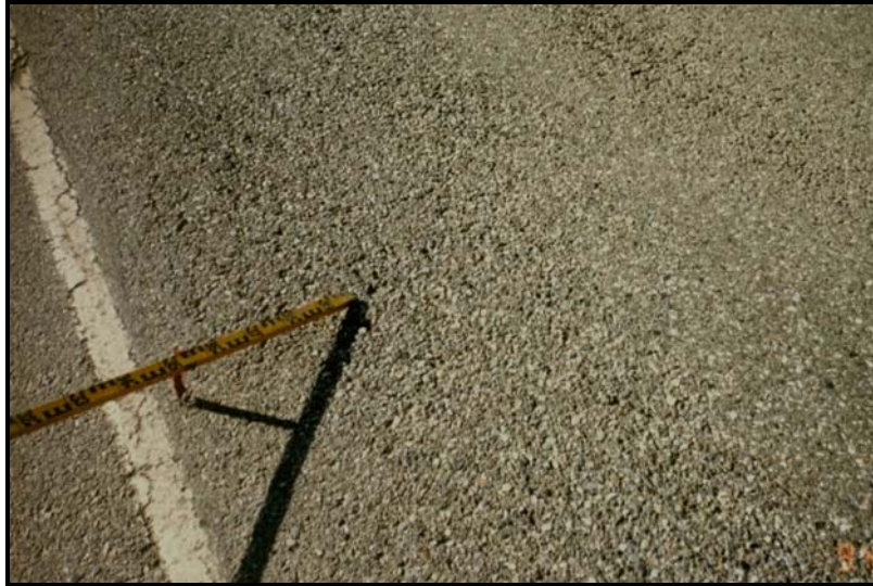
Figure 39 - Moderate Severity RAV
