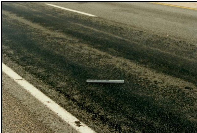
Figure 34 - High Severity BLD
