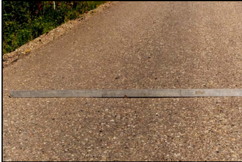
Figure 25 - Low Severity RUT
