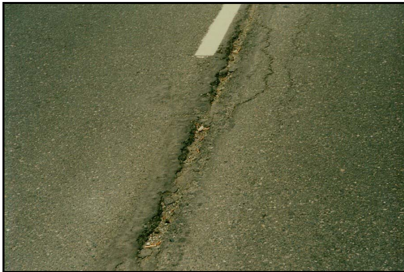
Figure 8 - High Severity LJC (single crack)
