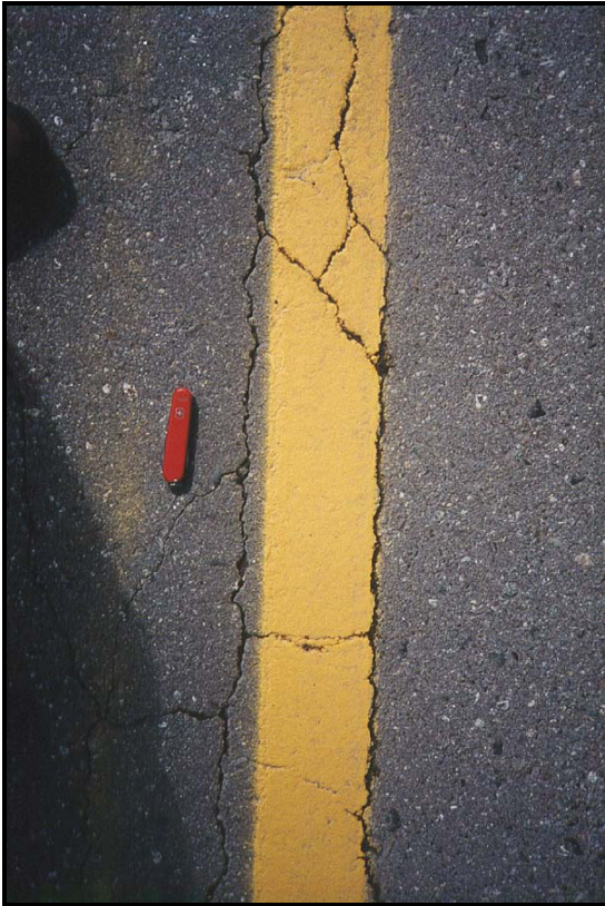
Figure 5 - Low Severity LJC
