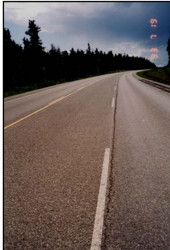
Figure 6 - Moderate Severity LJC
