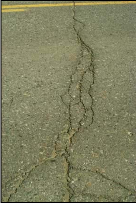
Figure 15 - High Severity TC (multiple cracking and spalling)
