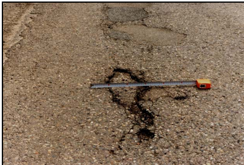
Figure 36 - Moderate Severity POT (close up view)
