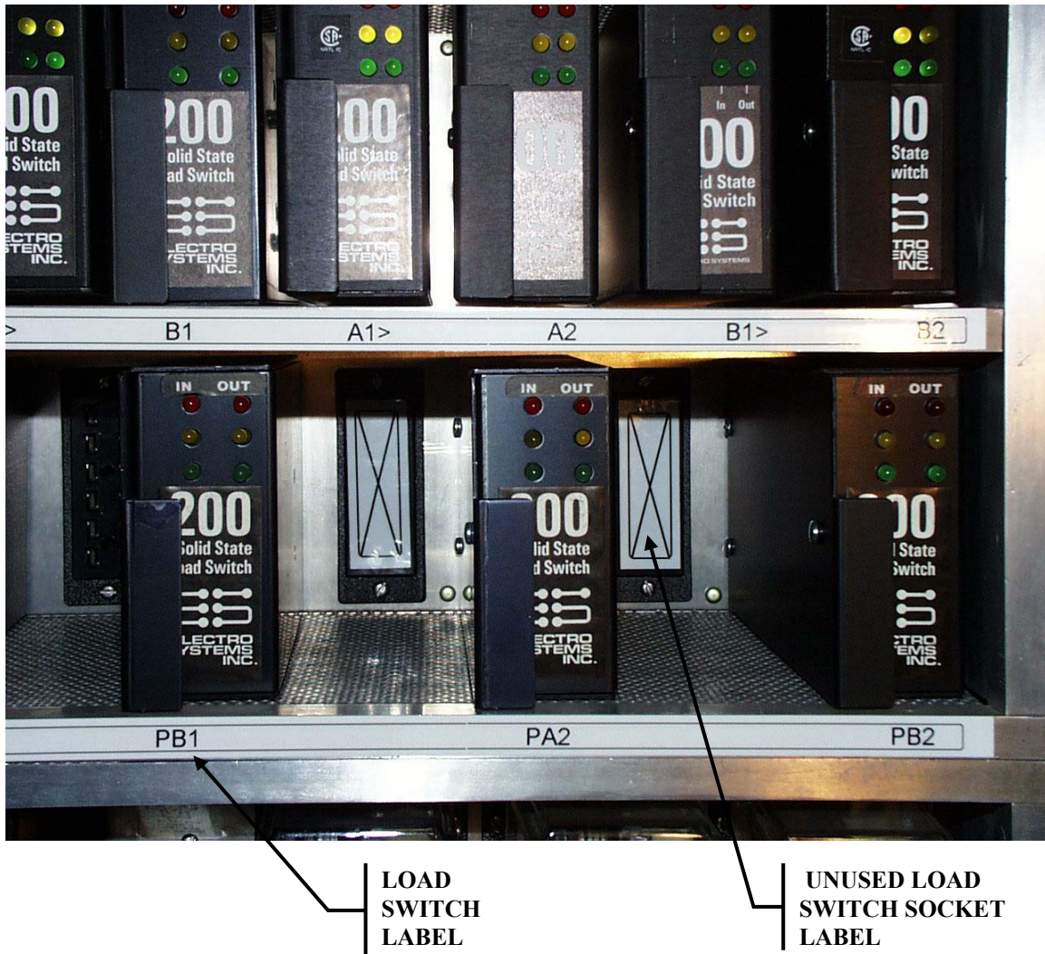
Figure 8. Typical Load Switch and Unused Load Switch Socket Label
