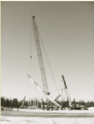
Above: Two cranes assist in the construction of the two flare stacks at an oil and gas facility.
