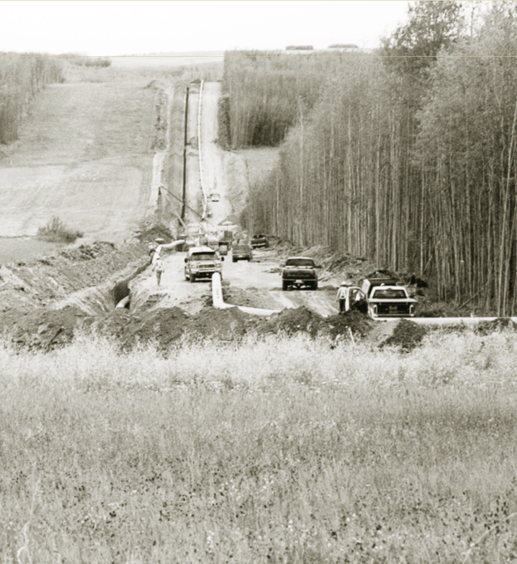
The OGC inspects oil and gas exploration, development and production in BC. Seen here is the laying of pipe during pipeline construction. Photo by Celia Hetrick
