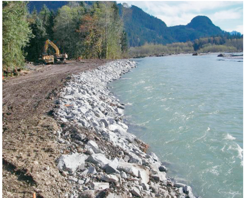
Swift progress is being made at the Pitt River site including the placement of erosion barriers.
