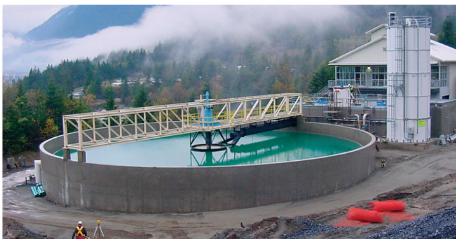
Britannia Water treatment plant clarifier.
