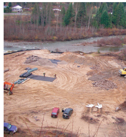
Tailings with rip-rap barrier being installed at Yankee Girl. Ymir is visible in the background.
