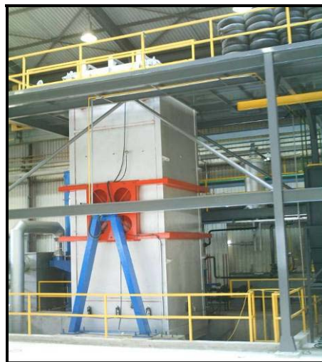
Figure 4.2.9 Low-temperature Conversion Pyrolysis Unit
