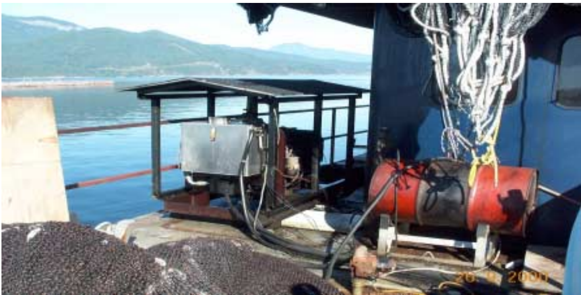
Photo 3. Generator Set (and fuel drum supply) without 110% containment.
