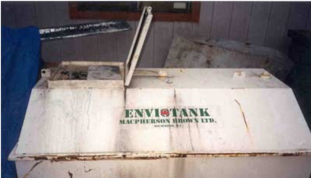
Photo 2. On-site fuel tank capable of 110% fuel storage containment.
