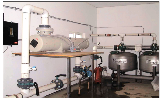
Figure 4 Ultraviolet Treatment Unit
