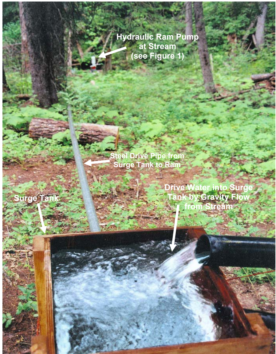
Figure 4 Surge Tank Supplying Drive Water to Hydraulic Ram Pump
