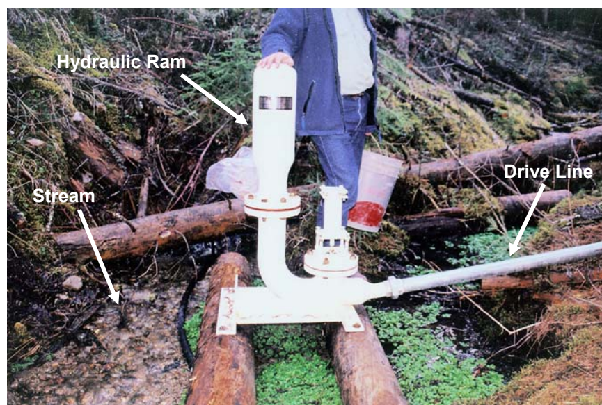
Figure 1 Hydraulic Ram Pump Installed Beside a Stream
