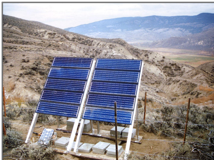
Figure 1 A Ten Panel Photovoltaic Array
