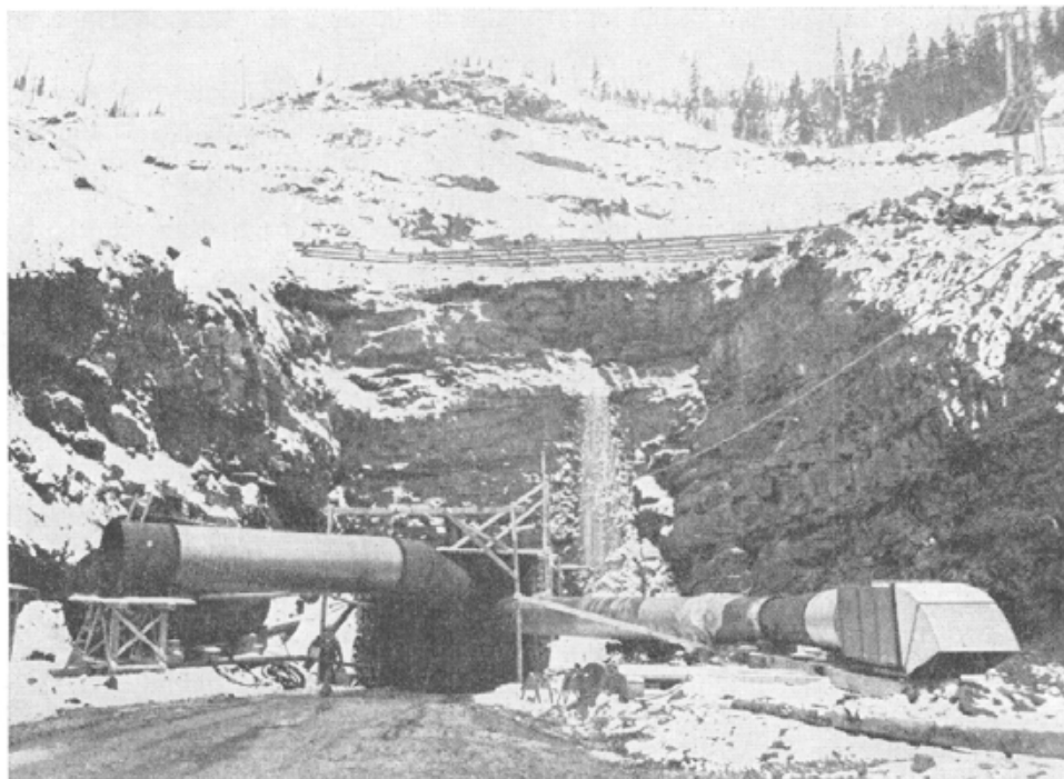
Plate VIIIb. Kaiser Coal Ltd., portal of the tunnel to be used for moving coal from the breaker station to the coal-preparation plant at Sparwood.
