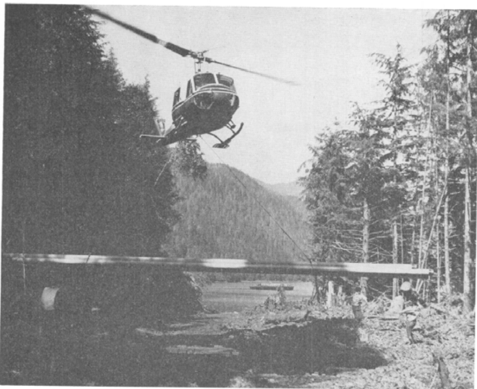
Plate IX. Helicopter stringing pipe along the Pacific Northern Gas right-of-way. (Courtesy of Westcoast Transmission Co. Ltd.)
