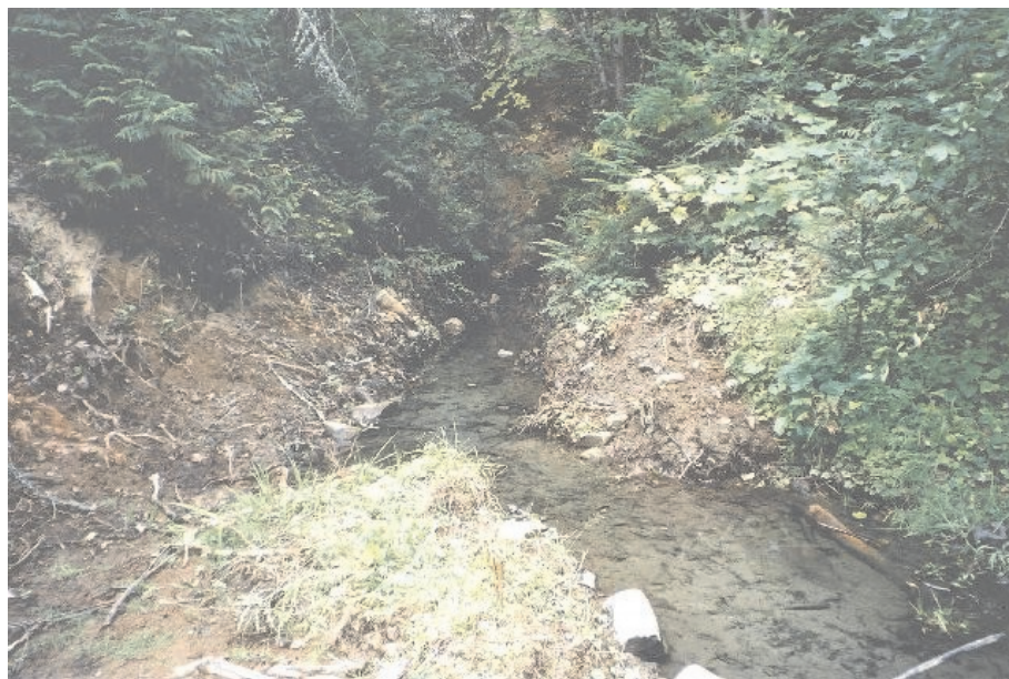
Photo 34. Portal backfilled with a culvert in place at the Gopher mine site. The drainage was sampled.
