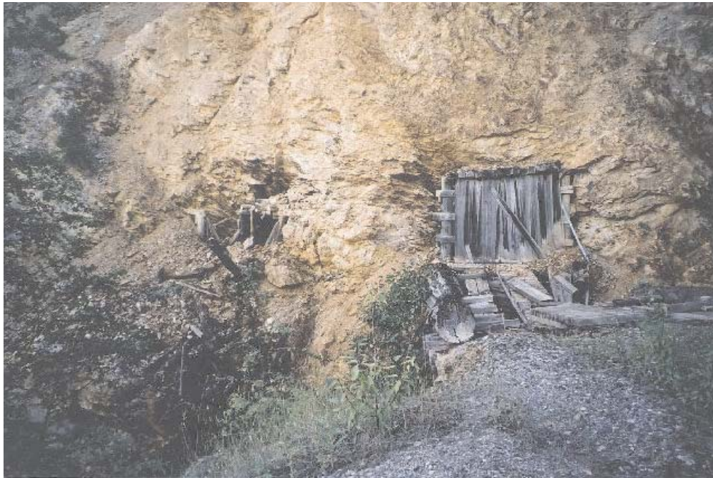
Photo 23. Homestake (Kamad) partially flooded upper adit. Homestake Creek flows beneath the bridge leading to the portal.
