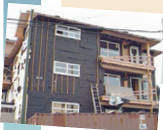
Photo courtesy of RDH Building Engineering Ltd.
