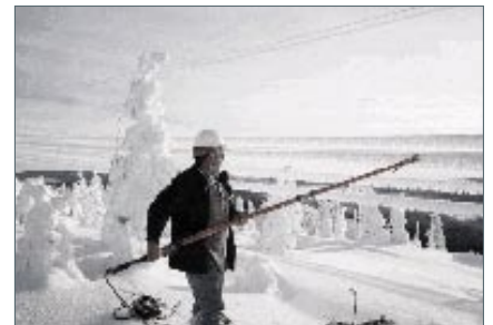
Unequal ice loading on transmission lines is one of the many challenges handled by the line maintenance team.
