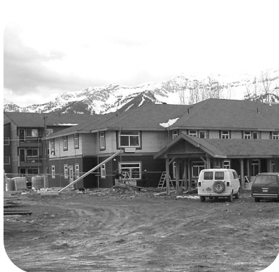
Rocky Mountain Village, a seniors' housing project in Fernie under construction in February 2004.
