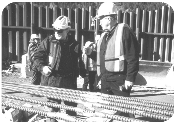
Minister Neufeld (right) met with the CBT Board of Directors and toured the Brilliant Expansion Project in March 2004. Picture above with Minister Neufeld is Mats Alexanderson, Project Manager for Brilliant Expansion Consortium.
