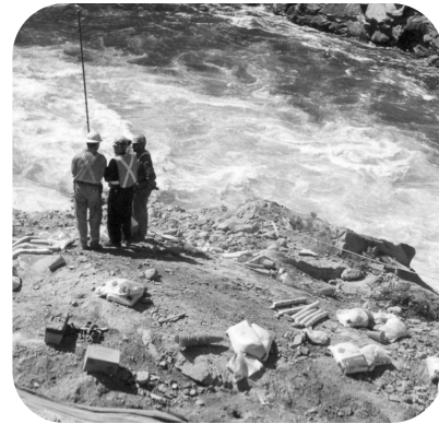
September 2003 - On site workers preparing for a blast at the Brilliant Expansion Project.
