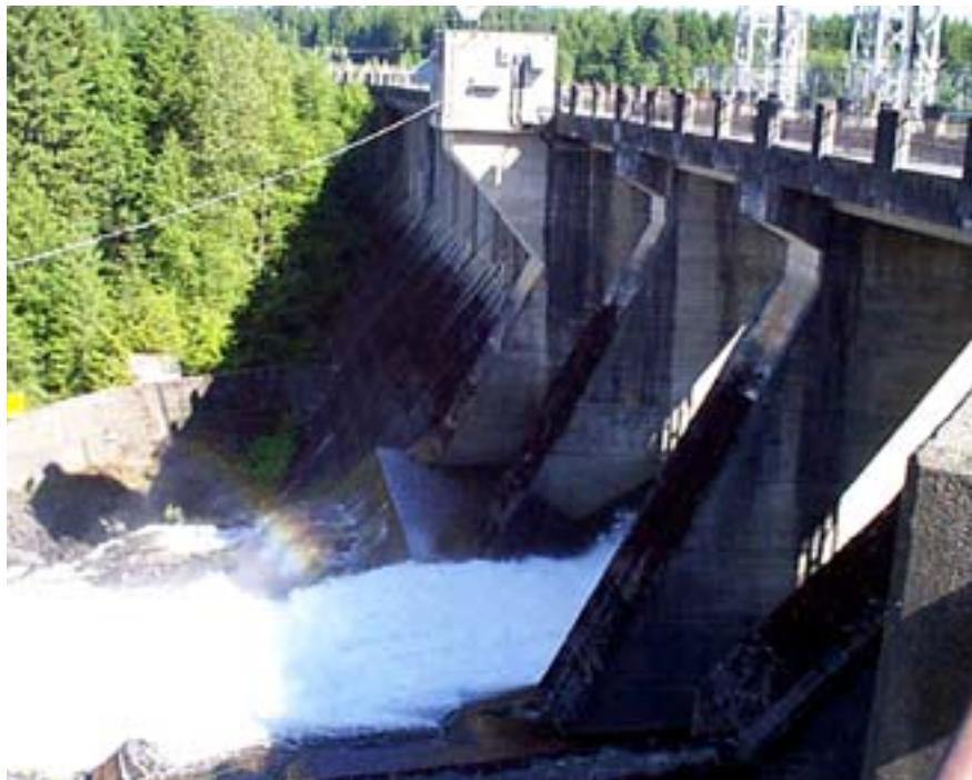
John Hart Generating Station is located on Vancouver Island and was originally constructed in 1953. Several options are being studied to address the condition and risk of the aging facility, including rehabilitation and redevelopment. Completion date is planned for 2010.
