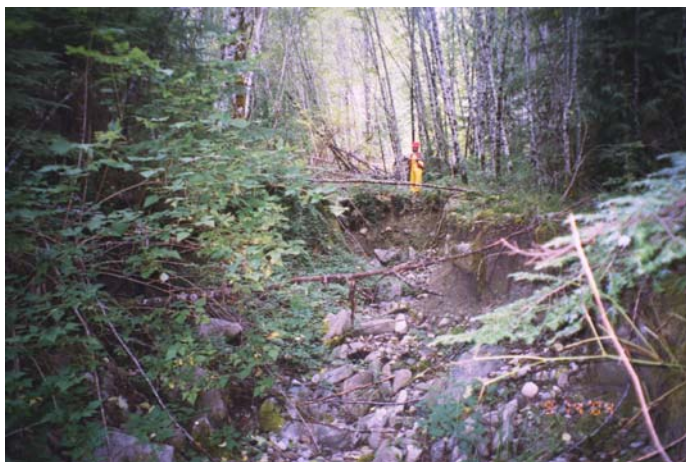
Figure 39. Deep knickpoint erosion along a climbing road that was caused by an avulsion that followed the road alignment.
