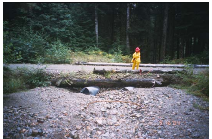
Figure 40. Road crossing of channel with naturally high sediment load (a wider box culvert would allow for better passage of sediment).
