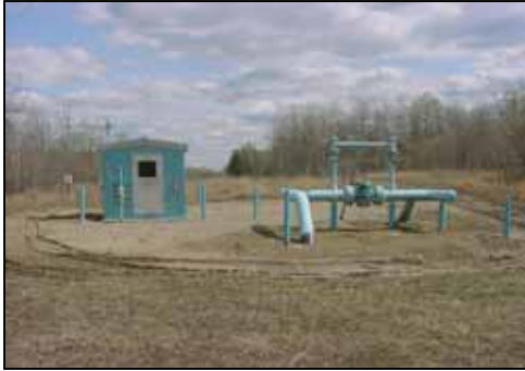
Photo #1 - Typical Natural Gas Metering Station
