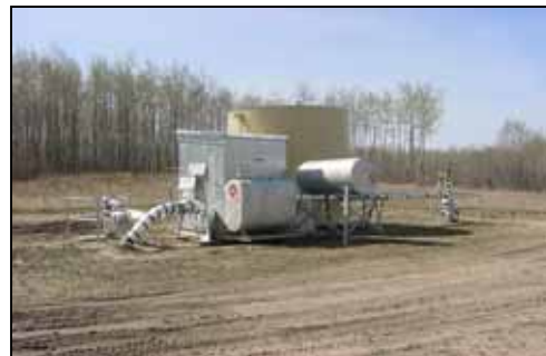
Photo #4 – Example of a Producing Natural Gas Well Site
