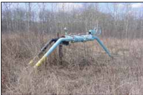
Photo #5 – Pipeline Riser
