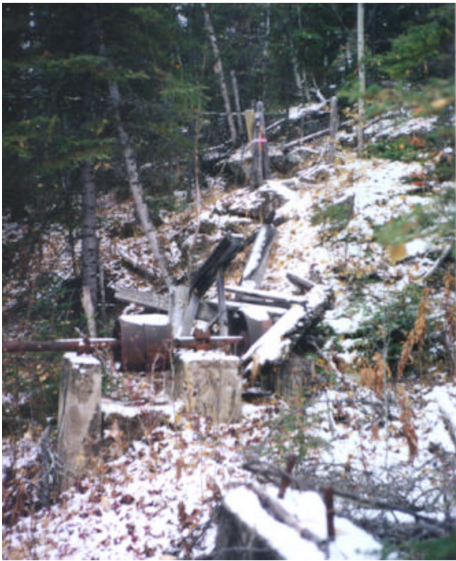
Photograph 6.7-4. Prince Albert Mine-Concrete Footings and Debris-October 18, 2002
