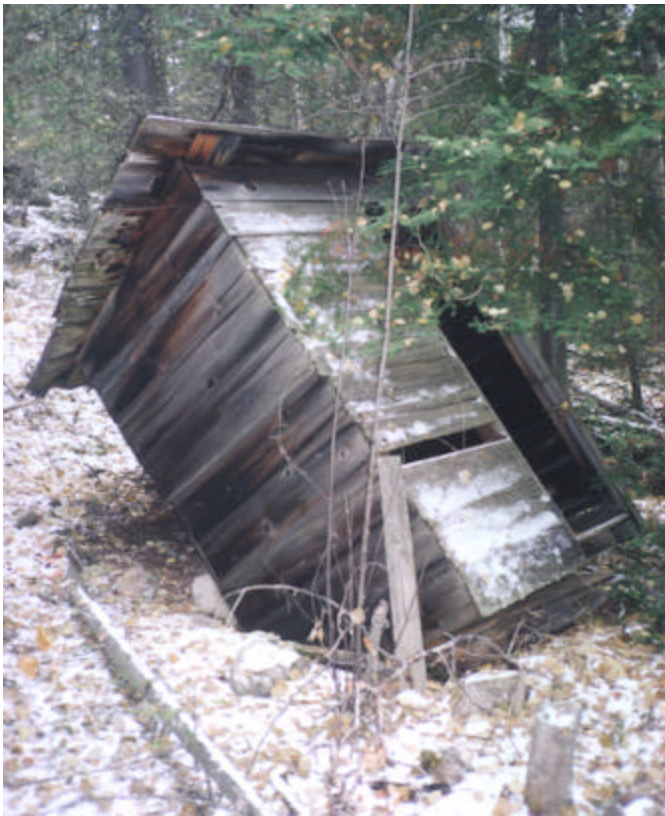
Photograph 6.7-6. Prince Albert Mine-Delapidated Building-October 18, 2002
