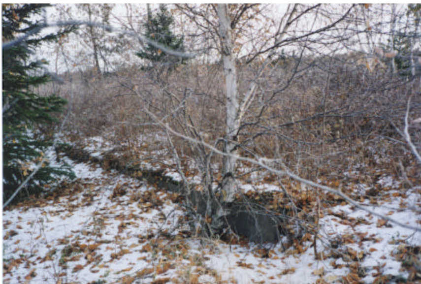
Photograph 6.18-6. Birch Lake Mine-Drainage Pipe-October 23, 2002.
