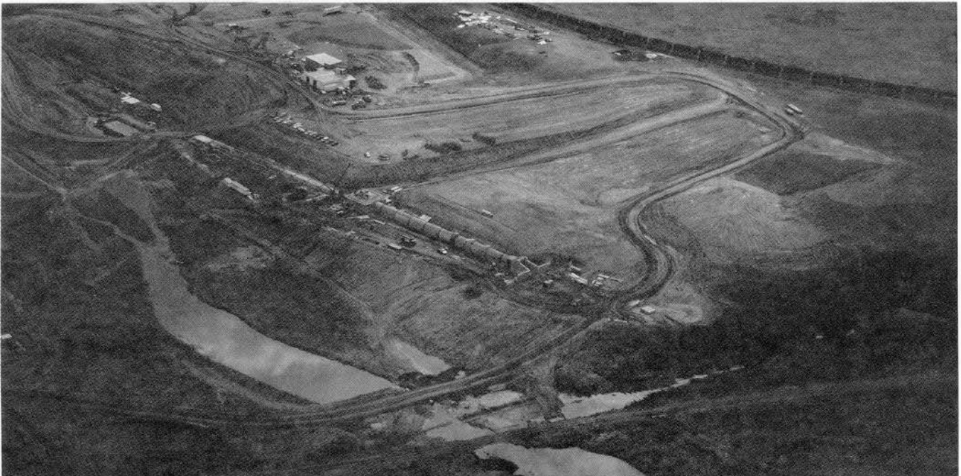
Alameda Dam construction site with the low-level outlet structure in the centre, April 1991 (photo credit: RJ Riewe)
