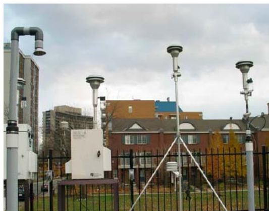
Figure 3 An air quality monitoring station
